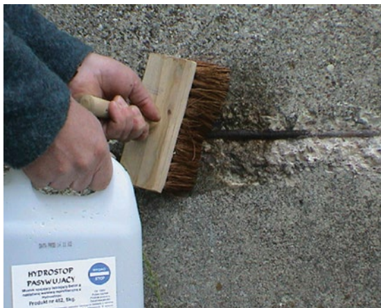
Fig. 1. Soaking concrete around a rod whose protective coating is not sufficient. After this procedure the surface will be reprofiled.
