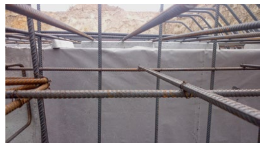
Photo. 2. Concrete being poured over a wall, with the surface covered with Penetrating Mat.
